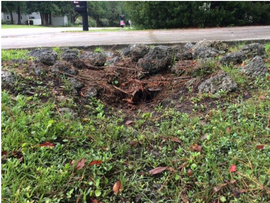
This is an example of a tile that is clogged with debris.
