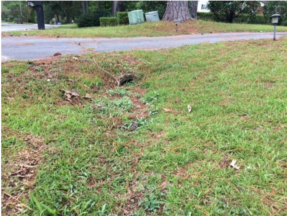
This tile is barely visible because it has become clogged with sedimentation over the years.
