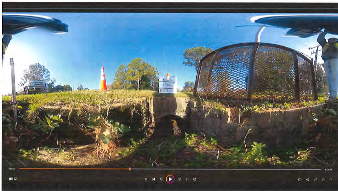
Node 10112 – Shoreline Drive Catch Basin
