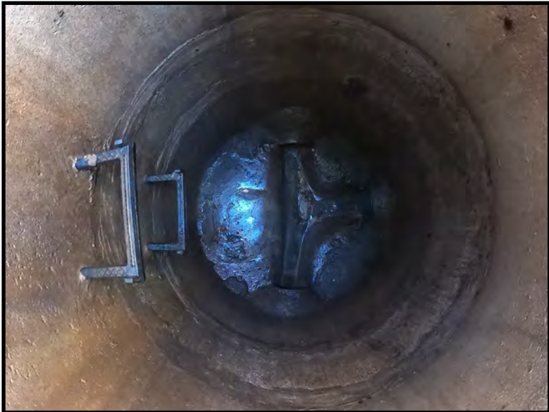
Typical Precast Manhole Interior
