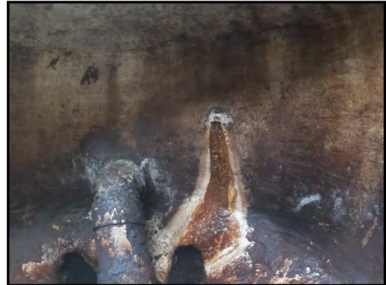
Hole in MH w/Soil Infiltration
