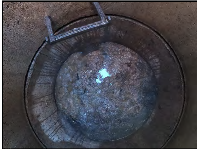
Backed Up Manhole
