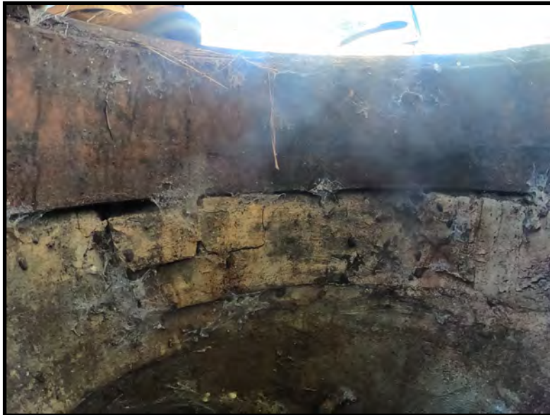
Manhole Frame Defects
