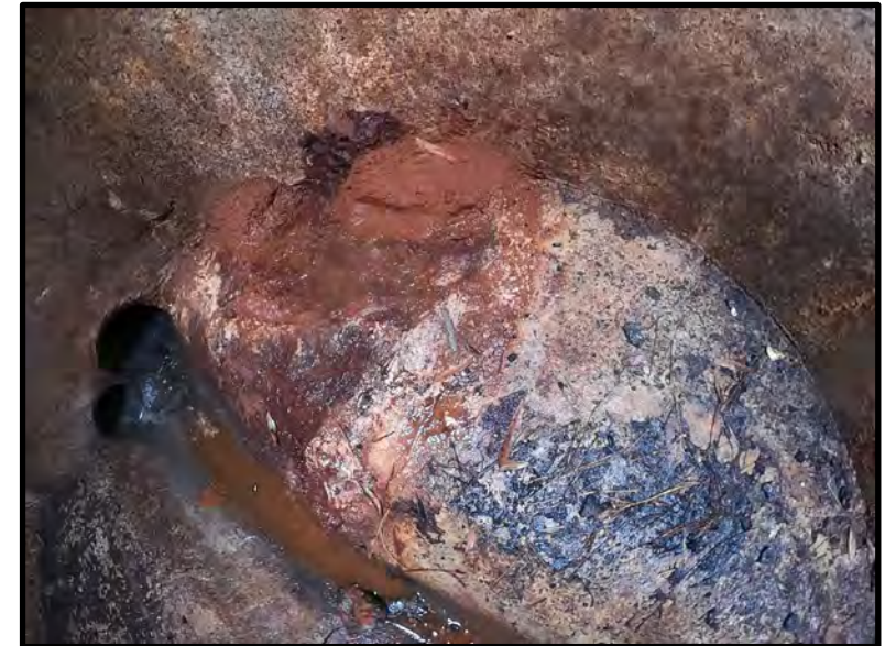
Soil Infiltration at Base of Manhole
