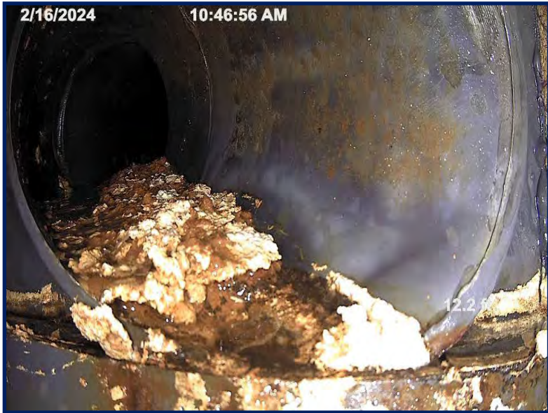
Debris Build-Up in Pipe
