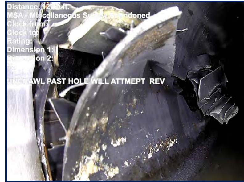
Structural Damage (cause unknown)
