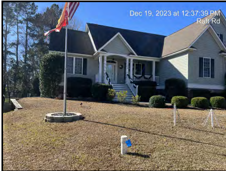
Leaking Clean-out Cap
