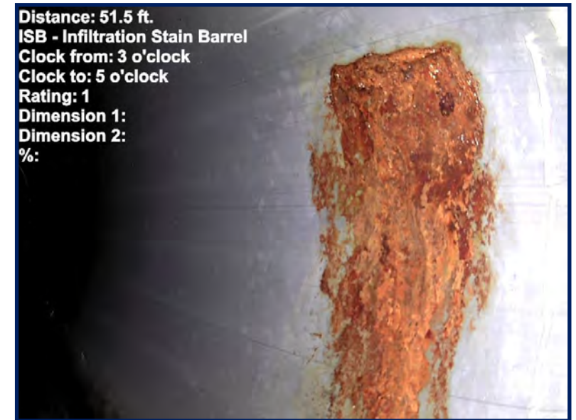
Pipe Wall Crack w/Infiltration Stain
