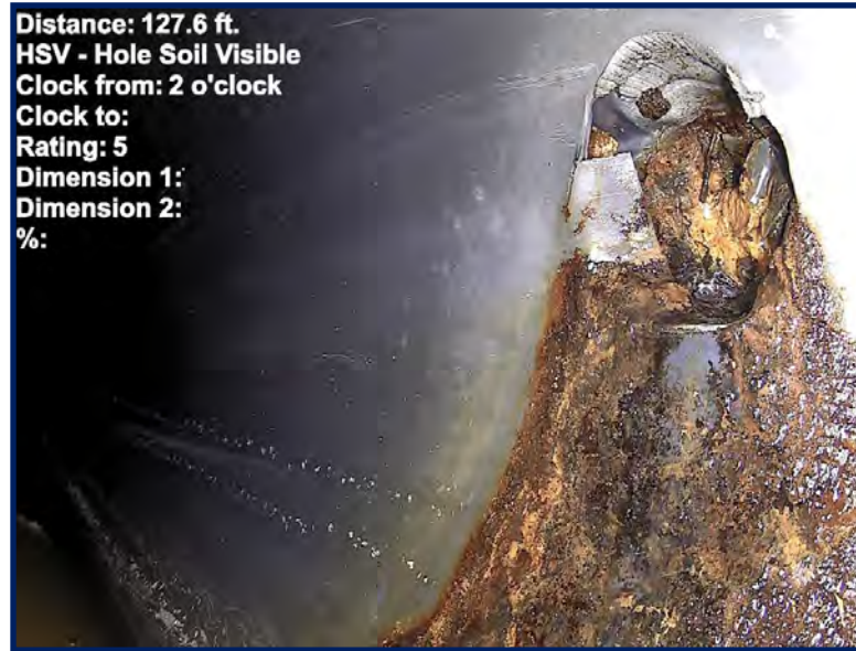
Hole in Pipe Wall (w/soi infiltration)
